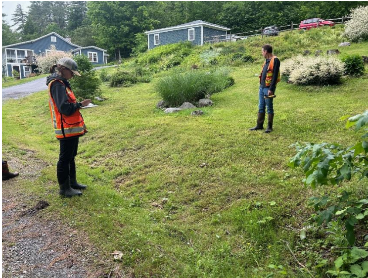
Photo 1: Project Lochlea Lane LL-01A – includes installation of a sediment forebay and bioretention basin in the grassy area located between the two FEA staff members.
