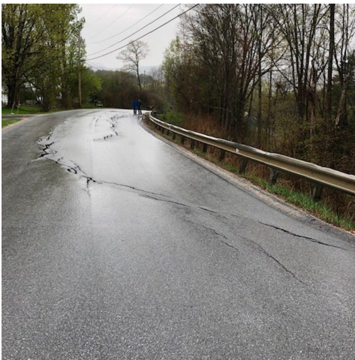
Dewey Avenue Cracking Due to Slope Failure
