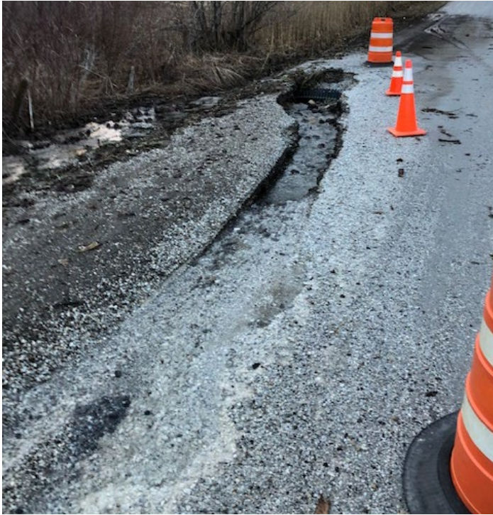
Flash Flooding on Marble Street
