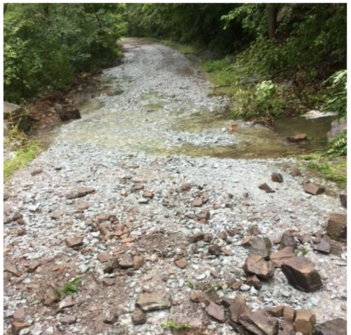
Flash Flood Damage on Gallick Road
