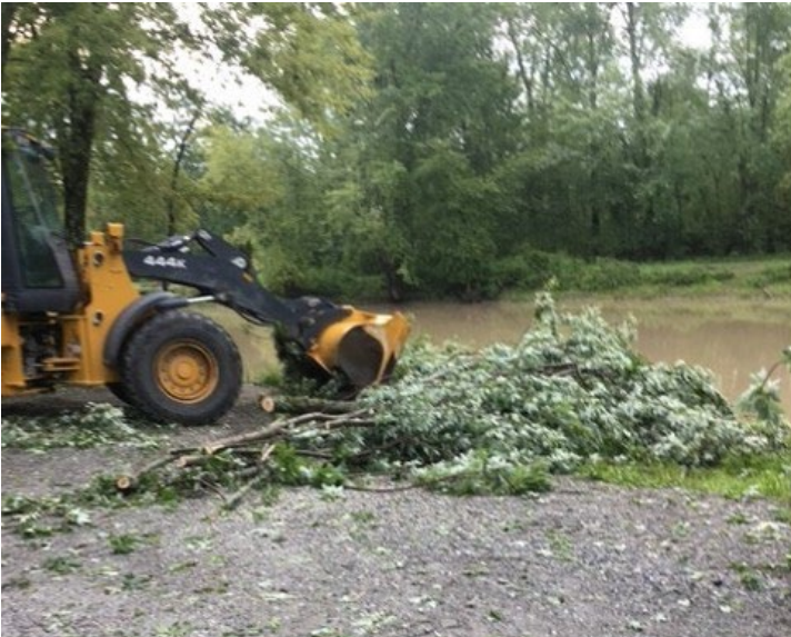
Debris Cleanup Following a Severe Storm on Gallick Road in 2020
