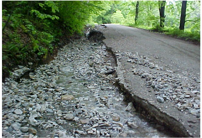
West Hill Road – July 2017 (DR4330) Storm Damage
