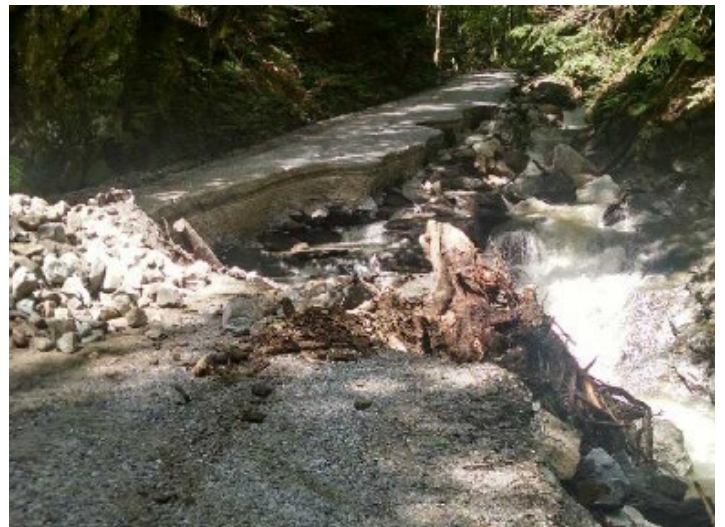
Dugway Road - July 2017 (DR4330) Fluvial Erosion
