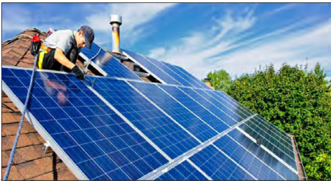
Courtesy: Rob Stubbins Solar Energy
