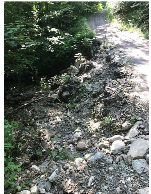
Flood damage to a road. Source: Bob Toppin.
