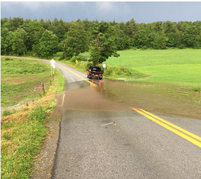
Inundation Flooding on VT Route 140 Near N East Road
