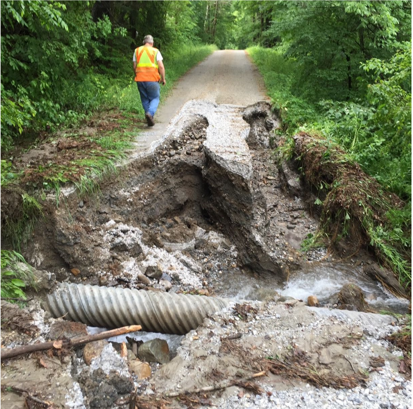
McCoy Road Washout – July 2017
