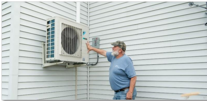
Rutland Town resident Fred Nicholson checking his heat pump. Courtesy: NeighborWorks of Western Vermont
