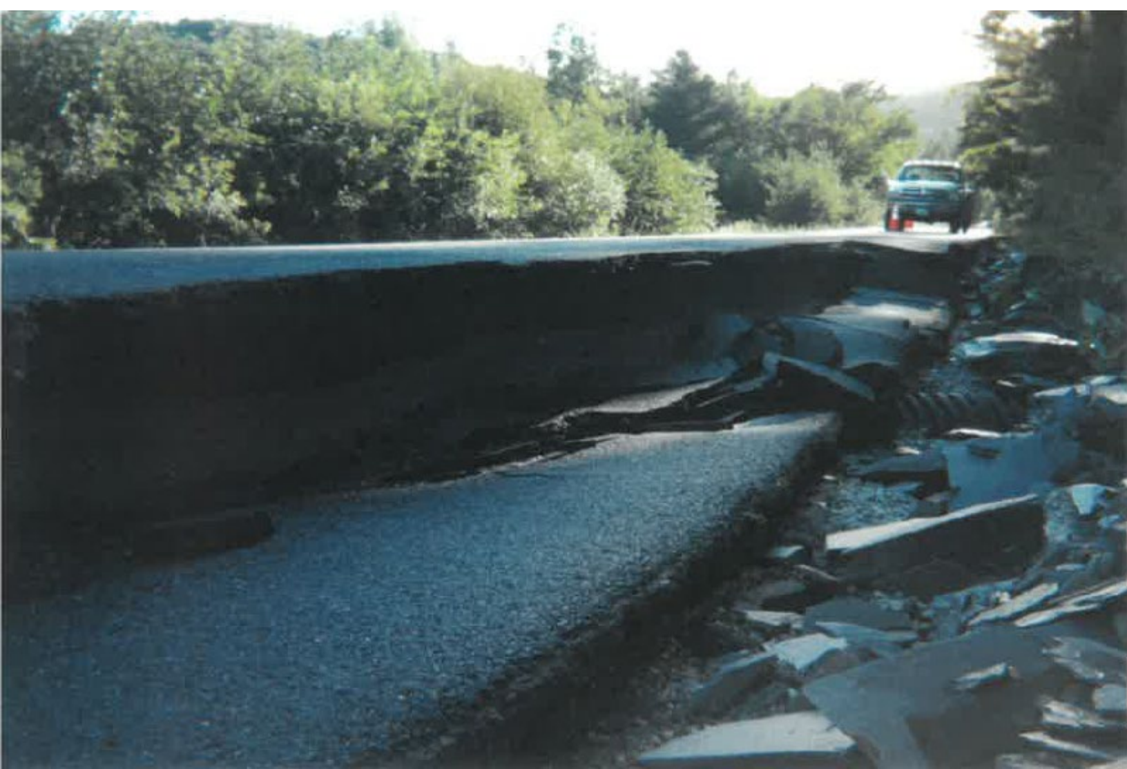
Partial Collapse of a Section of Monument Hill Road in August 2011 – DR4022
