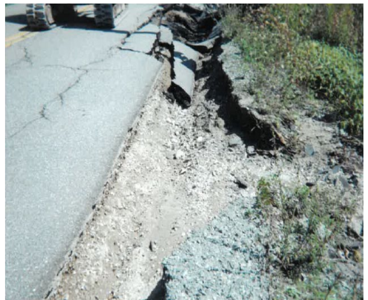
Shoulder damage on Monument Hill Road after Tropical Storm Irene (DR4022)
