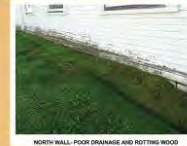
NORTH WALL- POOR DRAINAGE AND ROTTING WOOD
