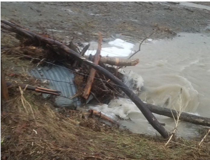
Piontek Road Plugged Culvert – April 2019
