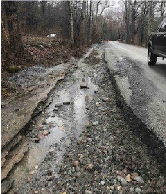
Belgo Road Flash Flood Damage – April 2019
