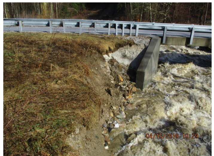
Fluvial Erosion Impacts to Bridge #25 over Mendon Brook on Medway Road – April 2019
