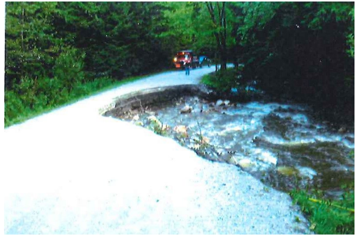
Flash Flooding Damage on Scottsville Road - 2017
