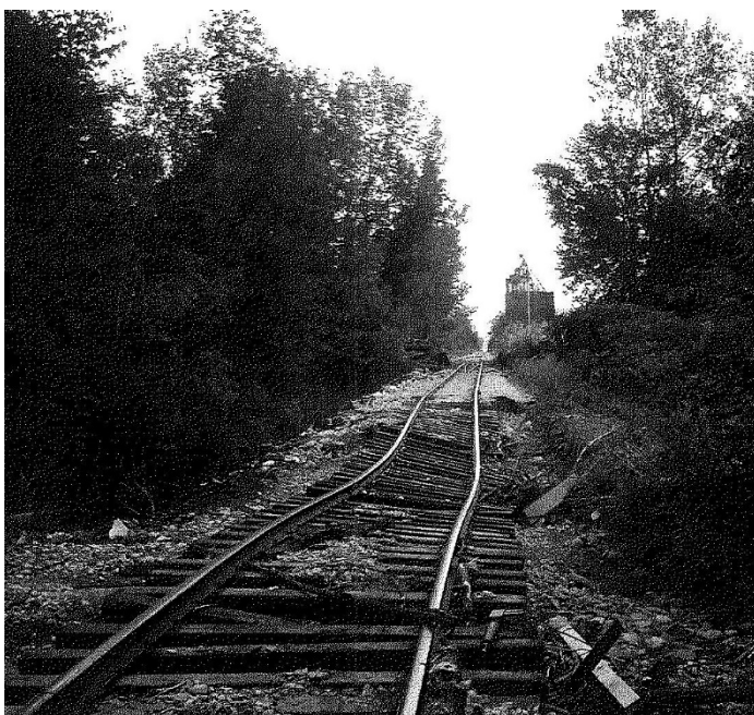
Railroad Track Damage from Tropical Storm Irene
