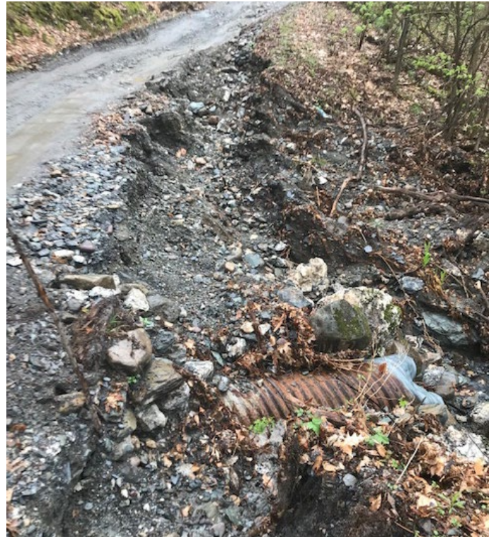
Flash Flooding Damage on Bird's Eye Road
