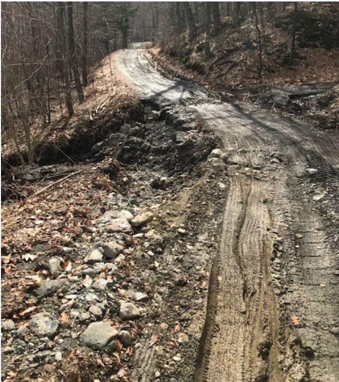
Flash Flooding Damage on Bird's Eye Road
