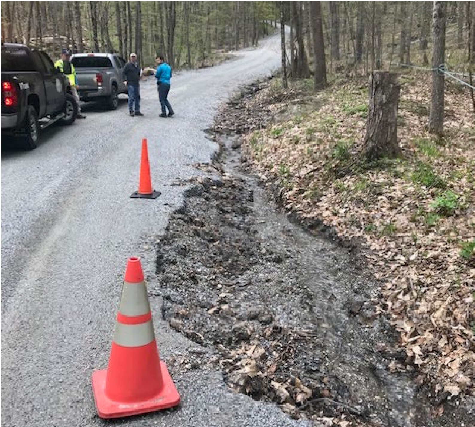
Pyka Road Washout – May 2019
