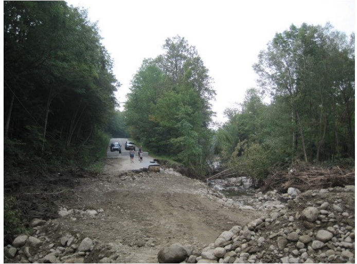
Irene Damages to Cold River Road
