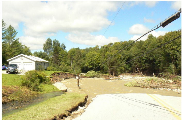
Irene Damages to Cold River Road
