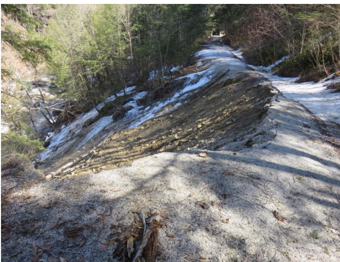
Cold River Fluvial Erosion along Upper Cold River Road
