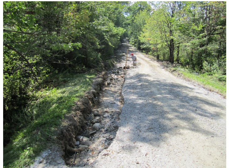
Flash Flood Damages along Eastham Road
