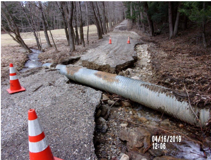
Goat Farm Road Perennial Stream Culvert Washout
