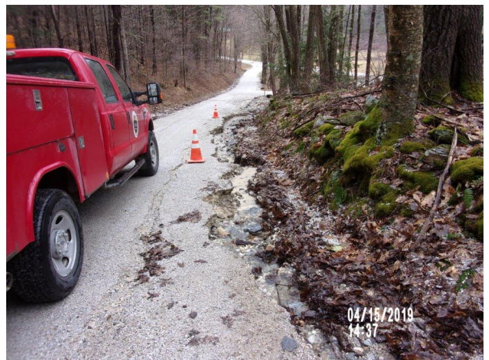
Allen Mills Road Flash Flooding Damage
