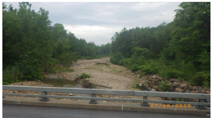
Gravel Deposition Upstream of B14 - 2020
