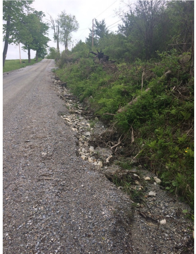
Flash Flooding Damage on Quarterline Road - 2019
