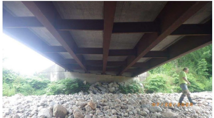
Gravel Deposition Under Middle Road Bridge (B14) on Cold River - 2020
