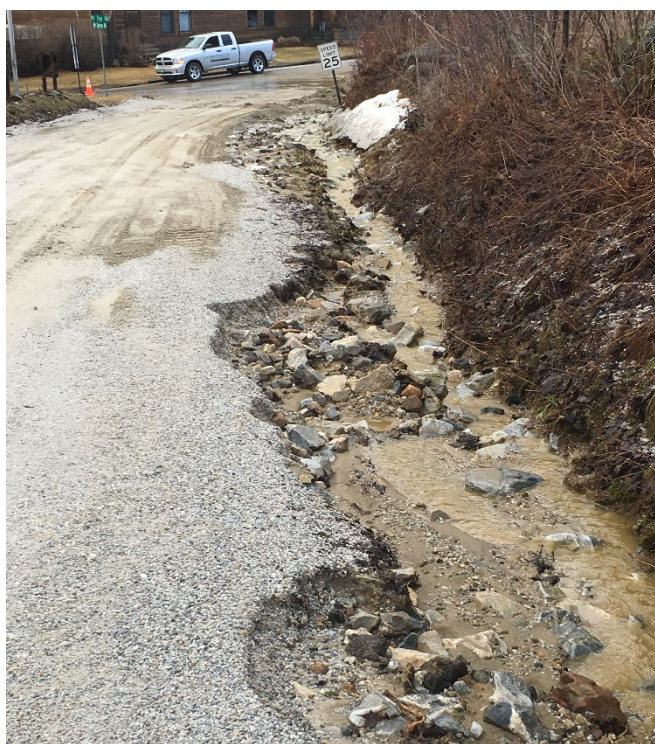
Flash Flood Damage on Mountain Spring Rd – April 2019
