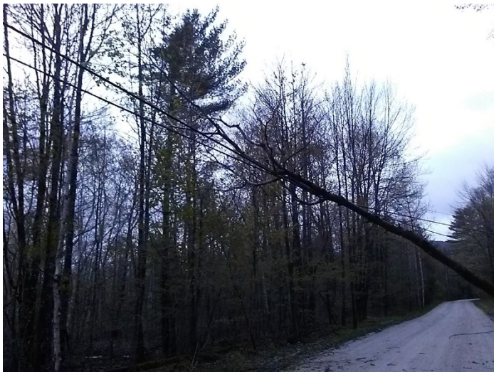
High Wind Damage – September 2017
