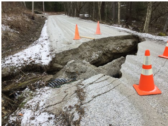
Flash Flood Damage on Mountain Top Road – April 2019
