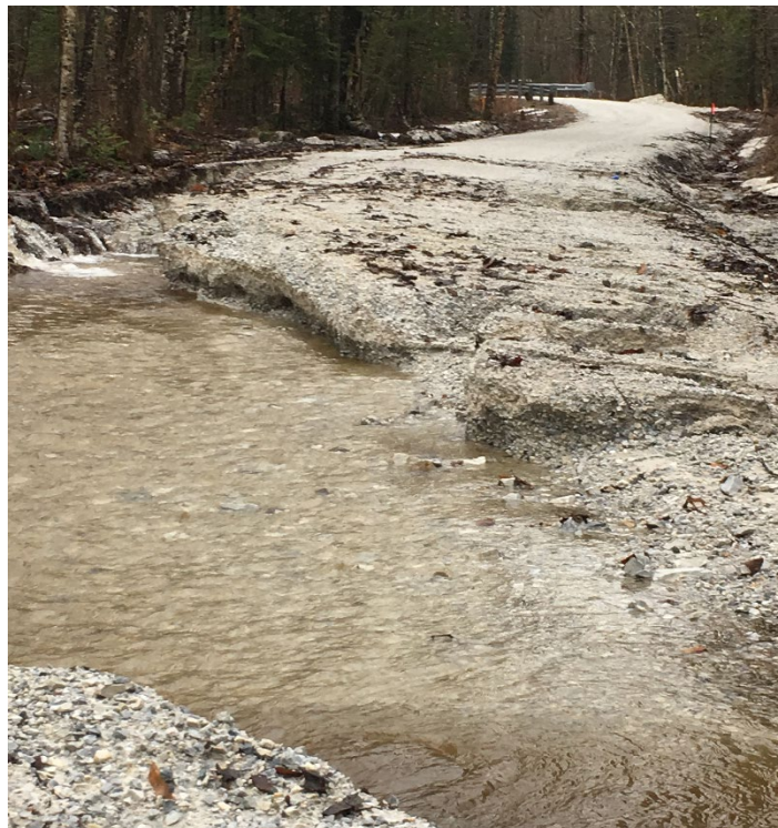
Inundation Flood Damage on Wildcat Road – April 2019 (Bridge 22 in background)
