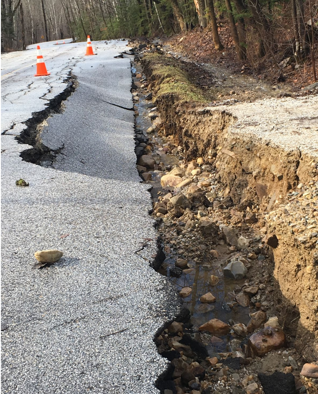
Flash Flood Damages on Mountain Top Road – April 2019
