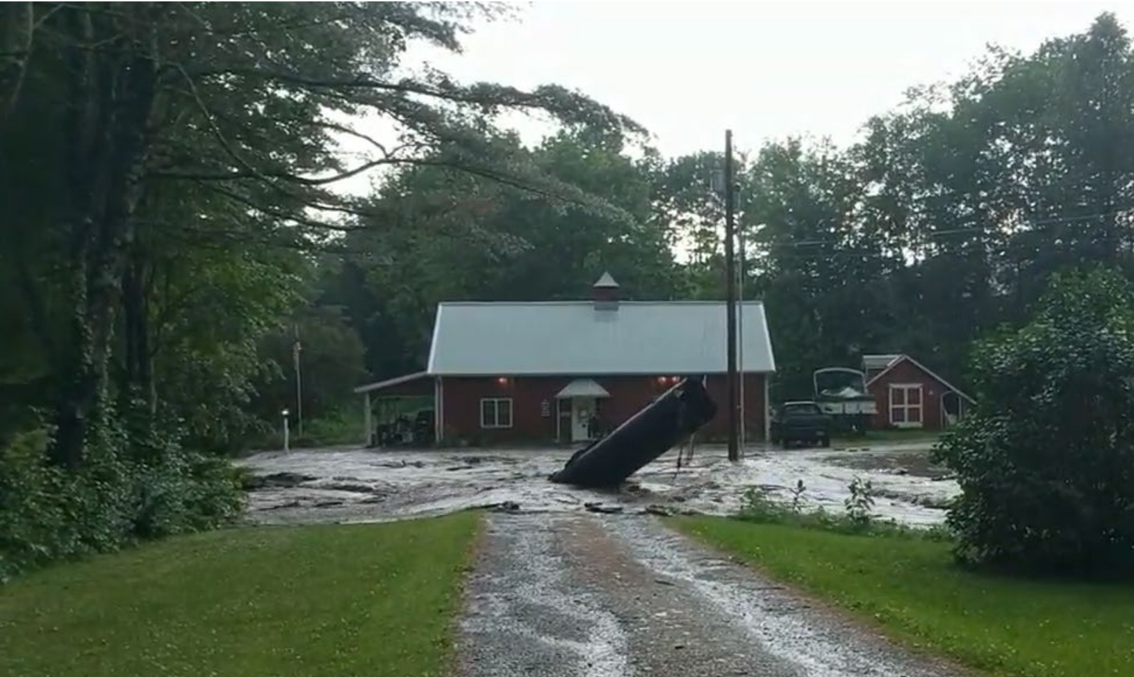
Culvert Washout on Capron Lane – July 1, 2017 Storm Event
