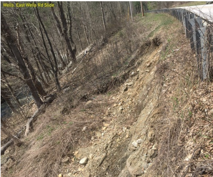
Approximately 200-foot long section of roadway on East Wells Road experiencing adjacent instability on a slope descending to Wells Brook.
