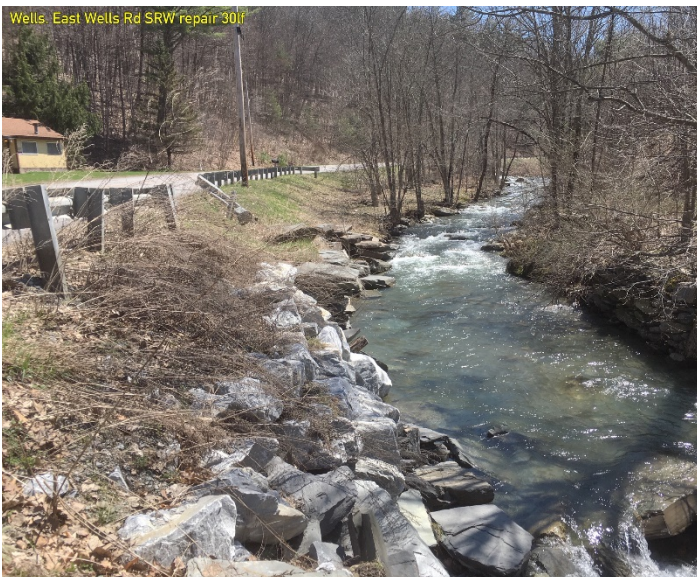
Approximately 30 linear feet of embankment subject to repetitive damage from flood events. Town installed a segmental retaining wall after Tropical Storm Irene and repaired it again in 2019.
