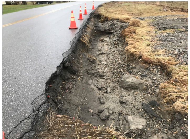
Inundation Flood Damage on Granville Street
