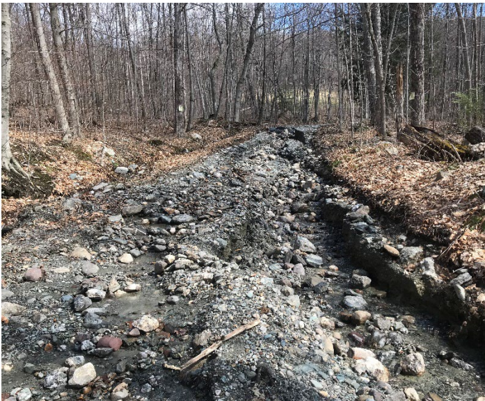
Flash Flooding on Ames Hollow Road
