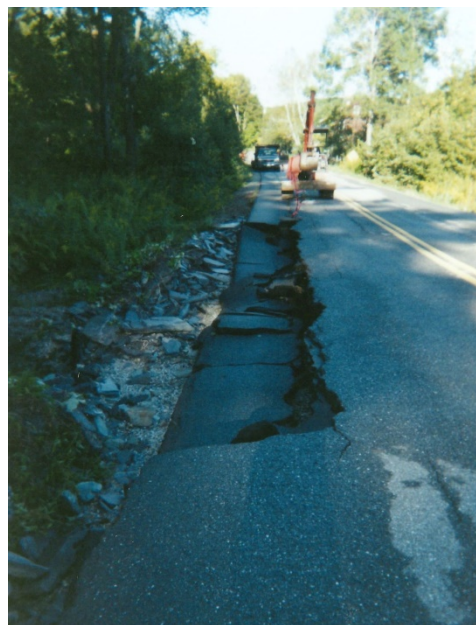
Monument Hill Road Washout - 2011
