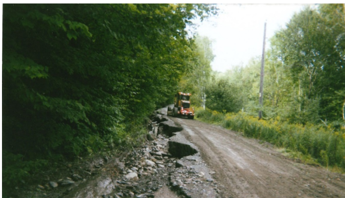
Ganson Hill Road E Washout - 2011
