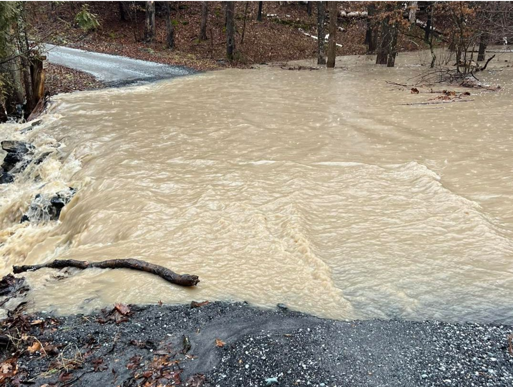
Stony Point Road Overtaken by Flash Flooding in December 2022 – DR4695
